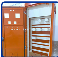
PANEL PDB HVAC
