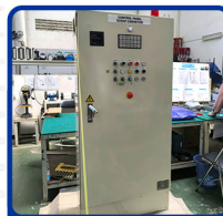
PANEL CONTROL SCRAB CONVEYOR
